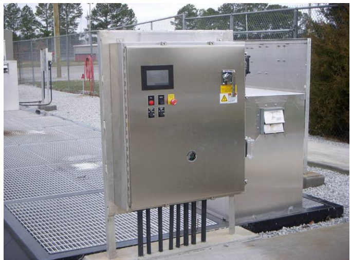
Figure 1 – Typical packaged system control panel
