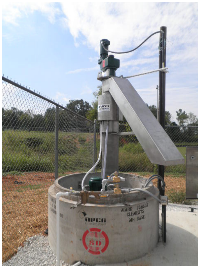
Figure 2- A sewage grinder is example of packaged equipment
